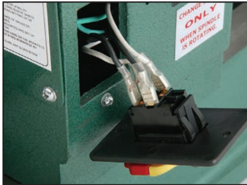
Figure 51. Paddle switch wiring.
